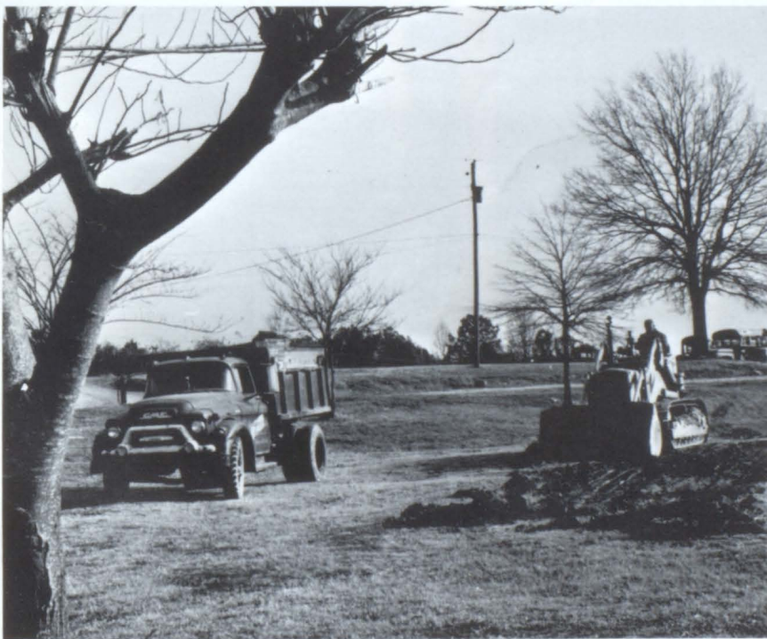
A dream becomes a reality - The Senior Class Project of 1970 gets underway.
